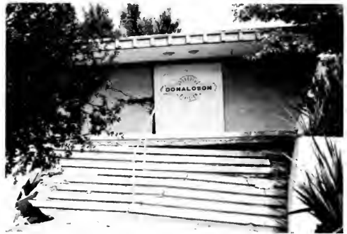
Photo 11. Arroyo light industrial tract. Damage to steps due to ground movement. E. G. Zacher photo.
